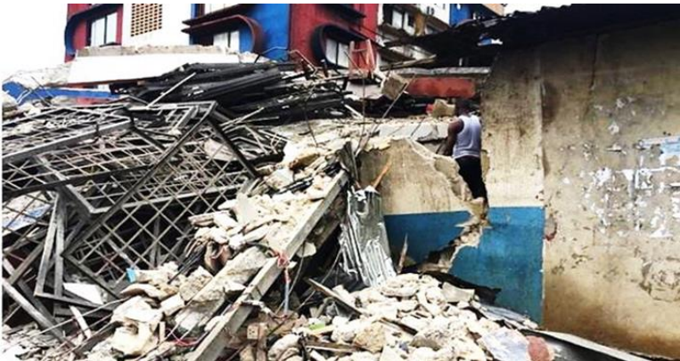
Fig 1.0: Collapsed school building at Rumubiakani
